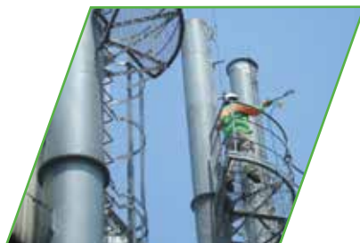
Stack Monitoring For Chimney
